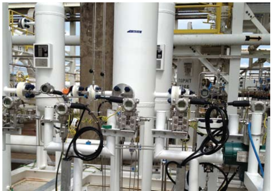
■ Onshore Gas Terminal in Kertih - Pilot Unit for Mercury Removal in Condensate
