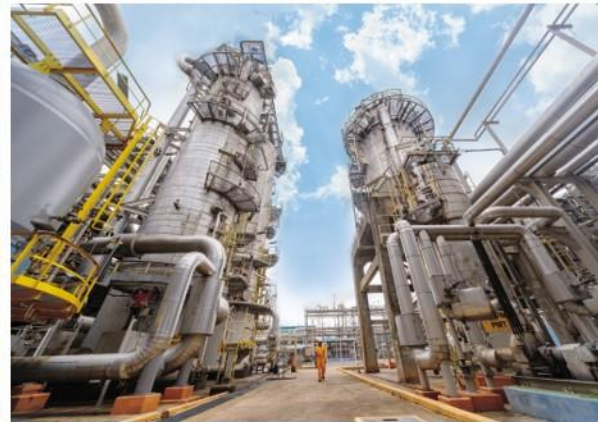
Uninterrupted gas supply
