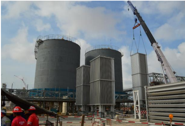
Storage tanks with capacity of 1,430 TPD oxygen and 780 TPD nitrogen
