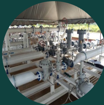
GTR Metering Station
